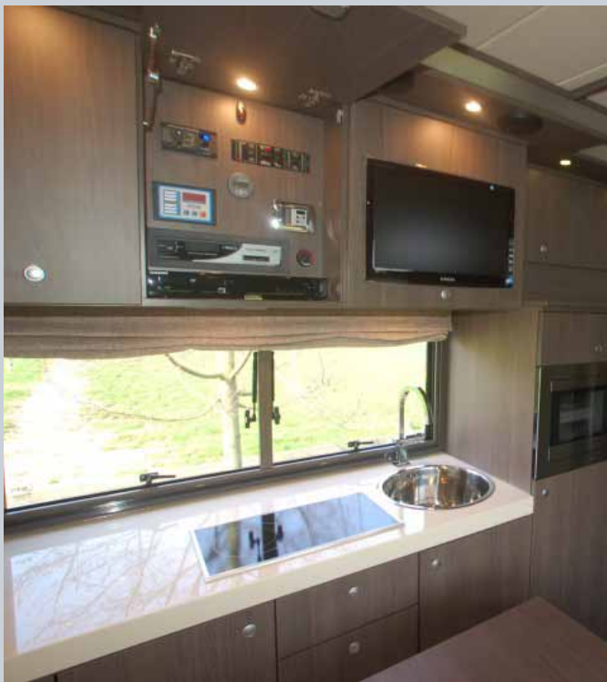
Photo 1: The BMV and the Digital MultiControl Panel from Victron Energy, installed in the horsetruck.
