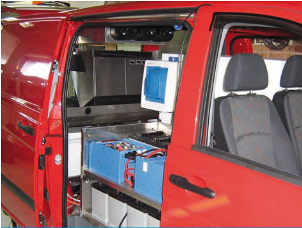
Installation of two paralleled Victron Energy MultiPlus 24/3000 inverter/charger units and battery bank.
