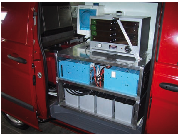
Two paralleled Victron Energy MultiPlus 24/3000 inverter/charger units and battery bank.
